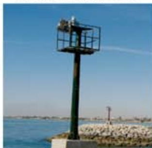
SL125/C lanterns mark wharf entrance, Bandar Abbas, Iran
